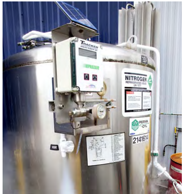
Permanent and transportable cryogenic tanks located at point-of-use
